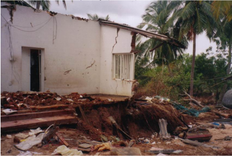
Photo 3. Damage to Kalametiya village (Dec 2005). Photo © S Senaratna Sellamuttu
