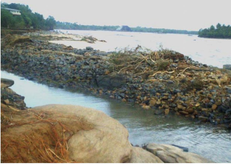
Photo 5. Kalametiya lagoon - damaged permanent outlet and breached sand bar (Dec 2005). Photo @ J Zietz
